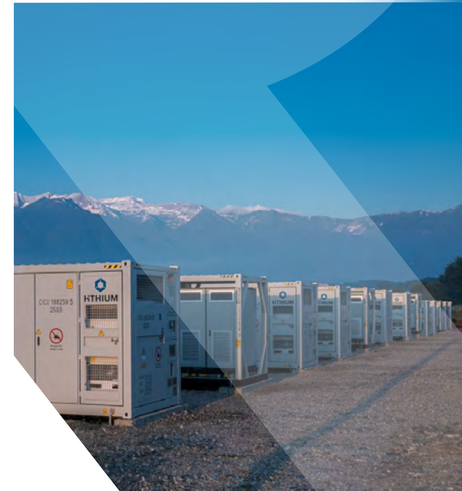
Storage of electricity, Renalfa, Razlog BESS, Bulgaria
