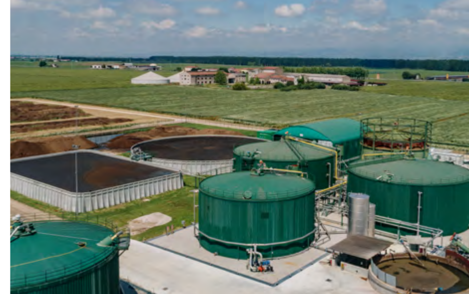
Biogas project, Belenergia, Ronco, Italy
