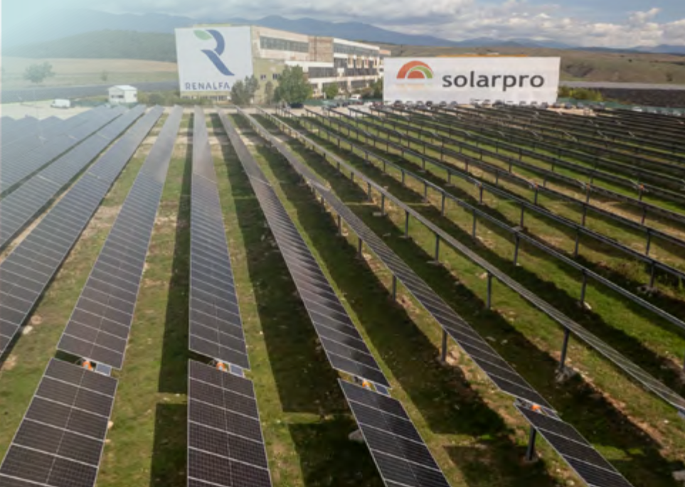
Photovoltaic solar project, Renalfa, Razlog, Bulgaria
